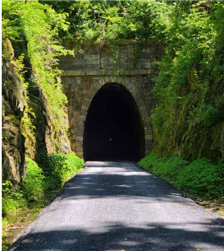
The west portal of the Blue Ridge Tunnel faces Augusta County.—Photo courtesy of Jack Looney.
